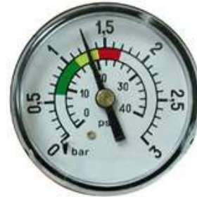
1,3 kg/cm 2 : The pressure is 0.5 kg/cm 2 more than the initial pressure, indicating that WASHING is required.
